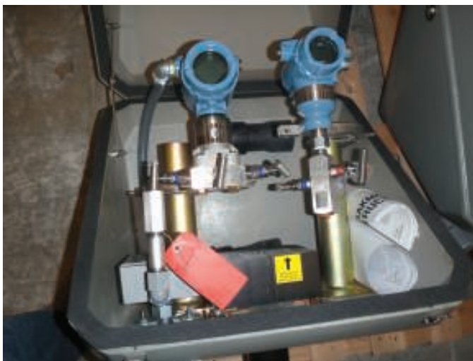
FIGURE 1. These pressure transmitters are connected to manifolds and mounted inside a sealed enclosure, which also contains thermostat-controlled heaters
